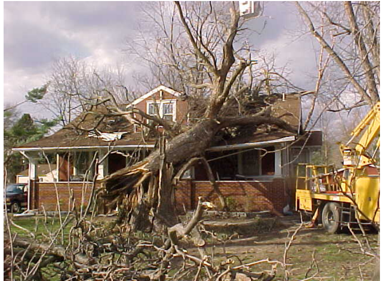
EXTENT OF DAMAGE INVESTIGATION
